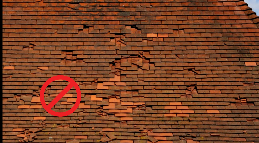
Damaged ceramic tile roof
